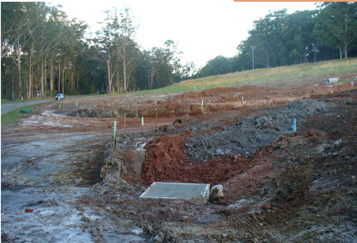
Example of poor sediment control on a building site. Photo K. Williams
