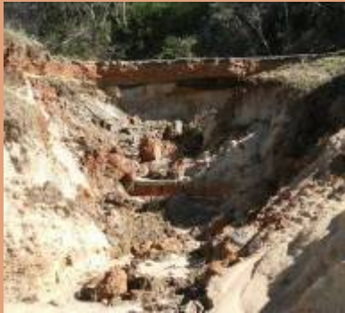
Erosion at Bellby's Beach Photo NSC
