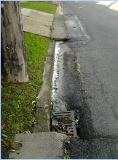
Pollution (paint) entering the stormwater System Photo NSC
