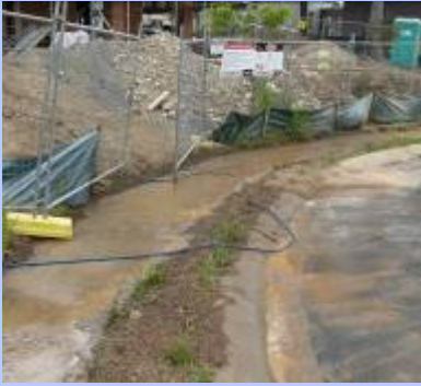
Pollution From a Construction Site Photo NSC
