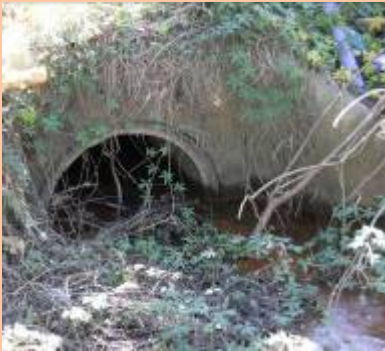
Dumped Rubbish Photo NSC
