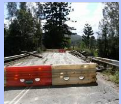
Flood Damaged Bridge, Valla Photo NSC
