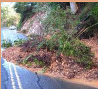
Land Slip on Riverside Drive Photo M Bryen
