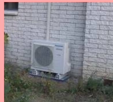
Air Conditioner Image Google
