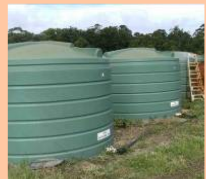
Leachate holding tanks Photo NSC
