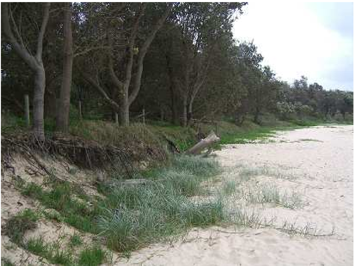
Figure A.9 – Top – Forster Beach car park (Block 2). Bottom – Forster Beach dune visible erosion (Block 2-3)
