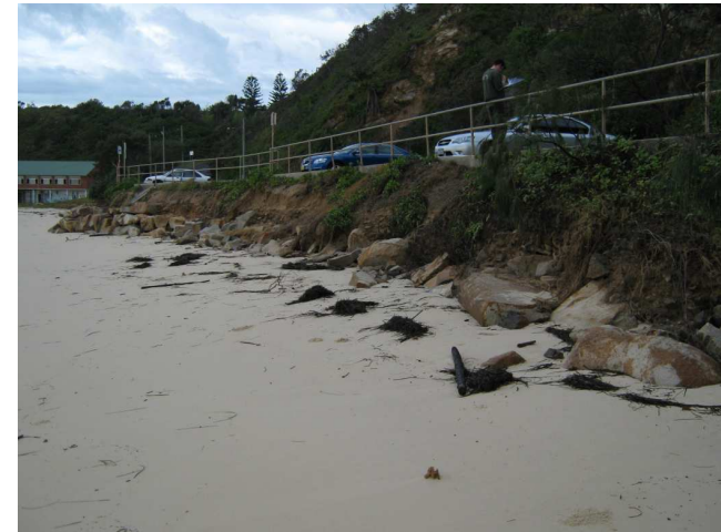
Carpark seawall, Main Beach May 28 2009
