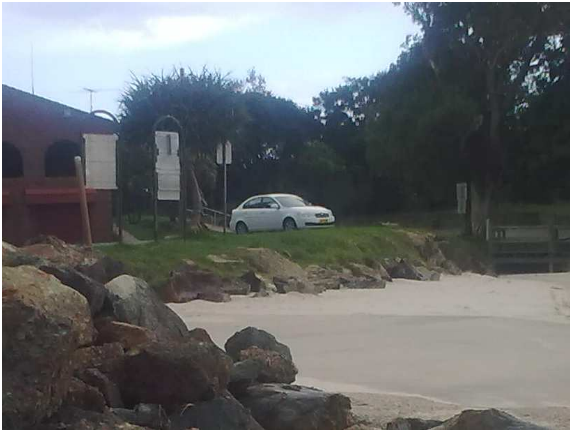
Figure 3.5 – Poorly built section of seawall, Scotts Head surf club
