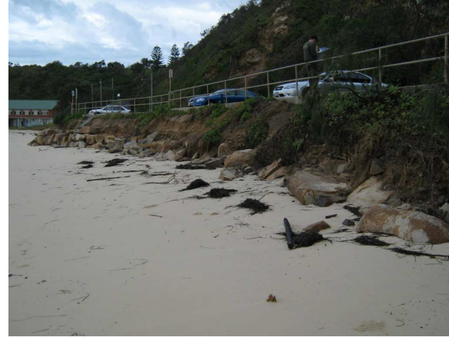
Carpark seawall, Main Beach May 28 2009
